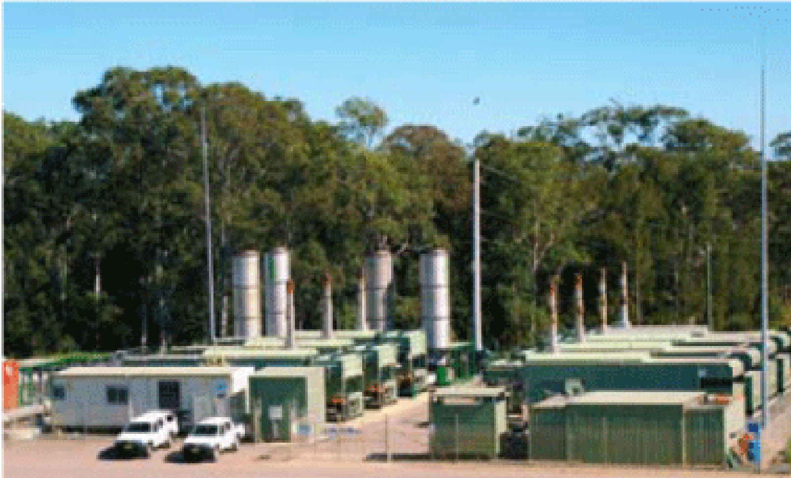
Landfill Gas – Eastern Creek (>5MW)
