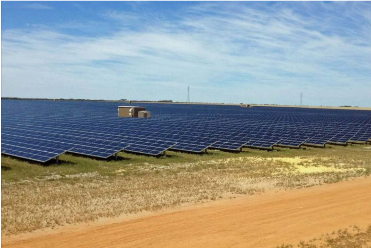
Greenough River Solar Farm (WA)
